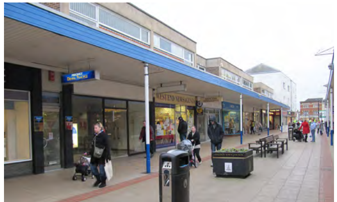
Fig 2.12 The canopy on Bury Street whilst providing protection from the elements can make the space appear dark and uninviting
